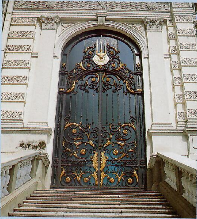
Door panels at the entrance to Chakri Maha Prasat made of iron decoratively wrought in beautiful designs.
